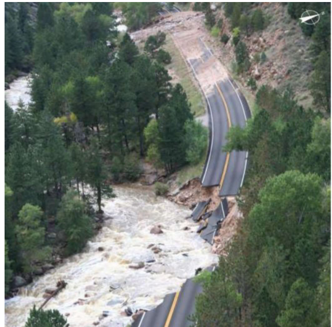
Exhibit 1.1: SH 7 (Lower) Middle St. Vrain Creek flood damage
